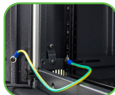
Front and rear doors equipped with ground wires
